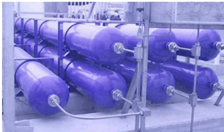
Storage vessels for Hydrogen, Design pressure: 450barg
